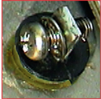
Epoxy has been added to a damaged key switch terminal insulator in an attempt to prevent accidental grounding.
