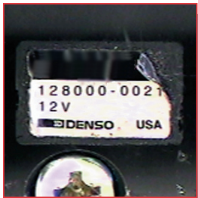
ID tag has been overheated and has shrunk. This is a sign of excessive heat.
