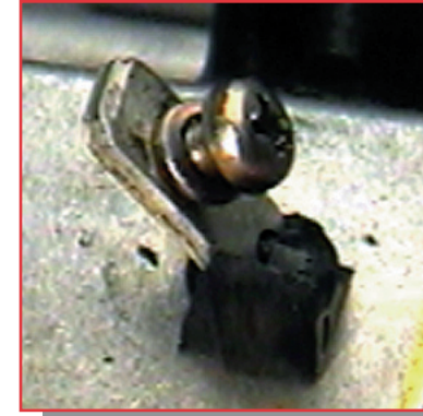
Key switch terminal insulator cover has been damaged. This terminal could possibly ground out on the starter housing.
