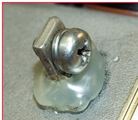
Epoxy has been added to a damaged key switch terminal insulator in an attempt to prevent accidental grounding.
