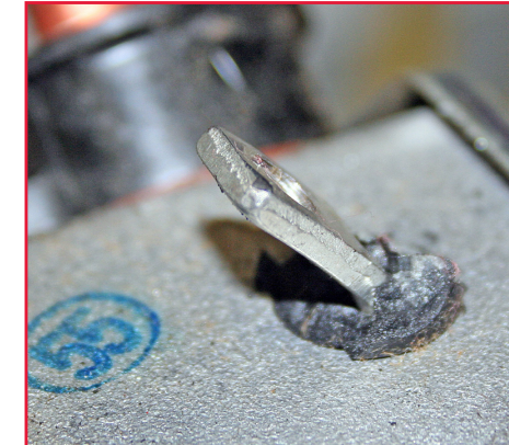
Damage to the terminal could cause ground contact with housing.
