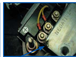
(E) Signs of Arcing
